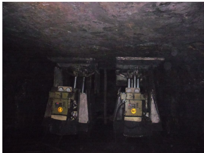
Figure 2: SAGES deployed for field trial at an underground mine in RK7 underground coal mine, Singareni Colliery Company Limited, India 2
