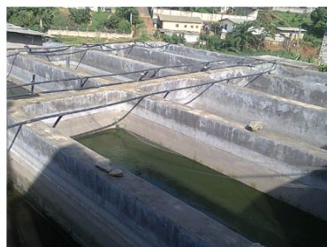
Plate 1 : Concrete fish ponds
