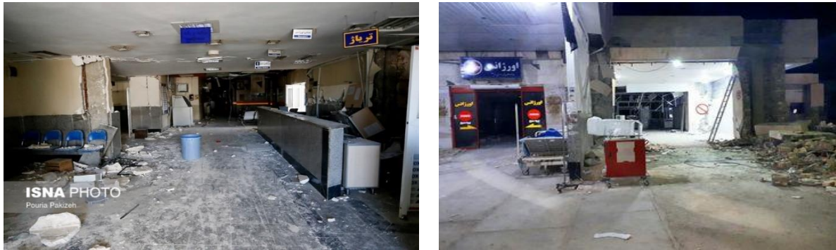
Fig. 1 The images of Imam Khomeini Hospital damaged after the Kermanshah earthquake in 2017
