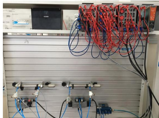
Fig. 42. Circuit designed on the electric stand.
